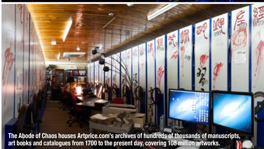
One of the underground server rooms, under the heliport, at the heart of the Abode of Chaos
